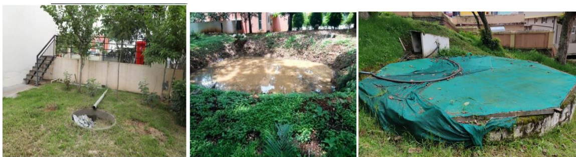
Rain water harvesting and retention facility in the campus
