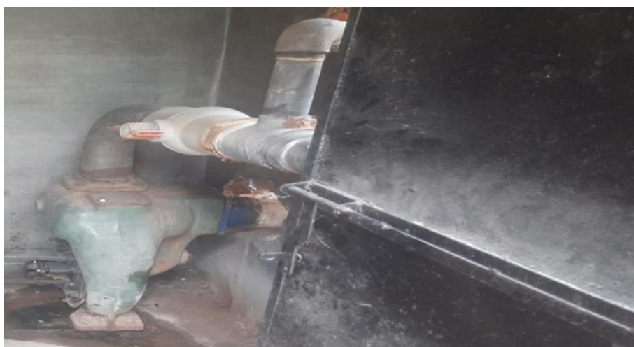
Pumps for disposing waste water into the sewage line
