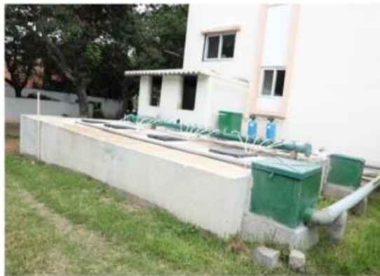
The small-scale sewage treatment plant
