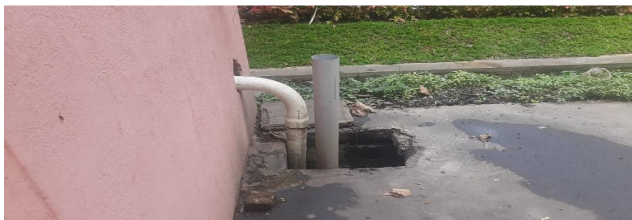
Storage tank (30,000 Litre)
