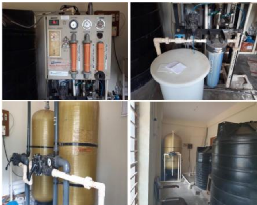
Facility for Reverse Osmosis (RO)
