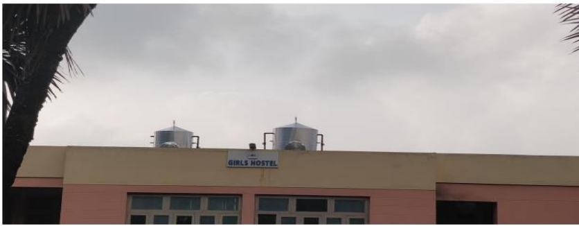
RO water facilities
