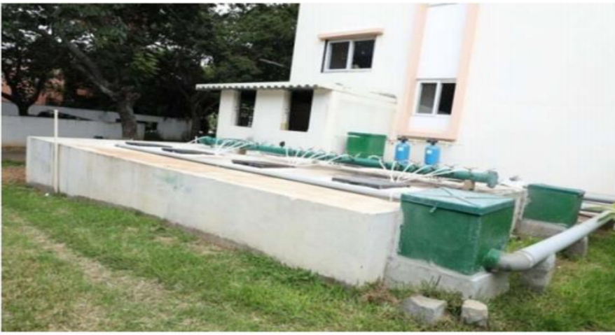
Small scale sewage treatment plant
