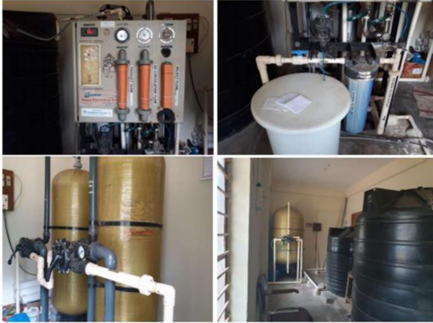
Facility for Reverse Osmosis (RO)
