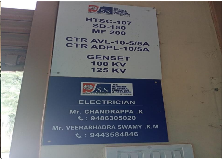
Electrical Control System
