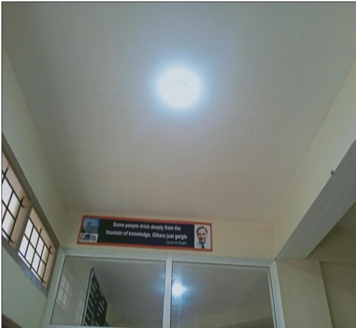
Energy Efficient LED Lights
