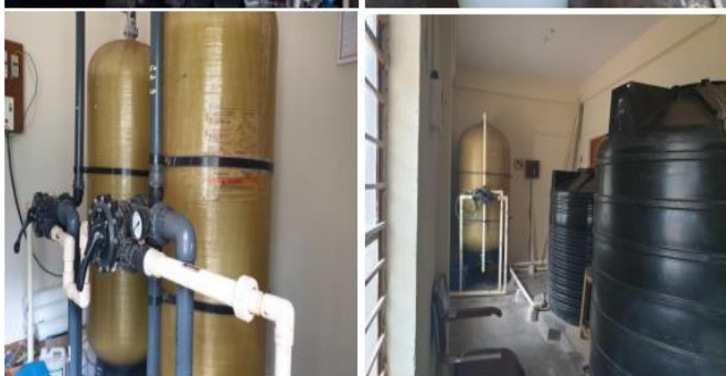
Facility for Reverse Osmosis (RO)
