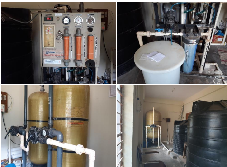
Current status of the RO Water Plant at the MCI
