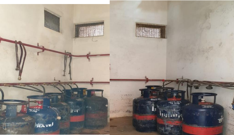
Centralised gas supply system
