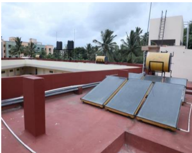
Solar panels at Hostels
