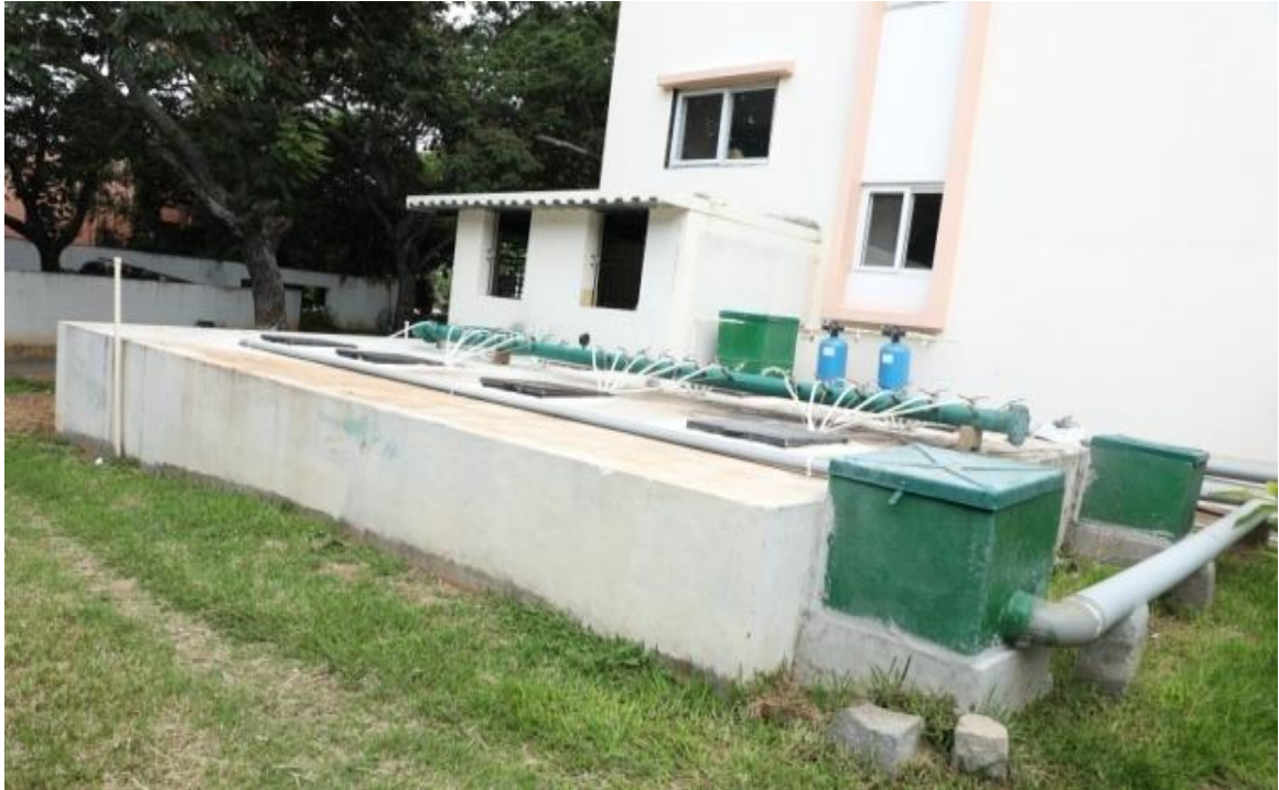
Existing small scale sewage treatment plant in the guest house
